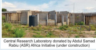
Central Research Laboratory donated by Abdul Samad Rabiu (ASR) Africa Initiative (under construction)
